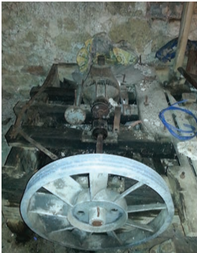
73. Motor mini-hidrocentrale – The engine of the mini-hydropower plant – Motor des Mini-Wasserkraftwerks
