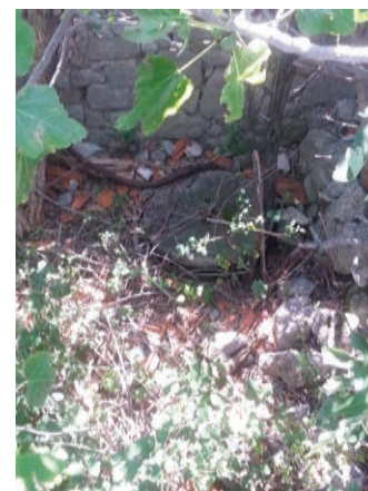
52. Zid i točak u Mandića mlinu – A wall and a wheel at the Mandića watermill Steinmauer und Mühlrad in der Mandić-Mühle
