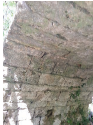
33. Sedreni krov Mlina kod Kudina mosta – A tufa roof of the watermill at Kude's bridge – Das Travertin-Dach der Mühle bei Kudin most
